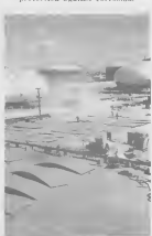
PRODUCTION LINE arrangement of metal sheets facilitates pre-assembly preparation. Sheets average six by eight feet and 12 1/2 sheets are required for erecting a 100mm-barrel tank.
